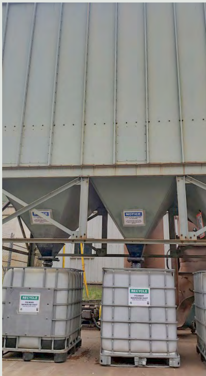
Baghouse dust collection system
